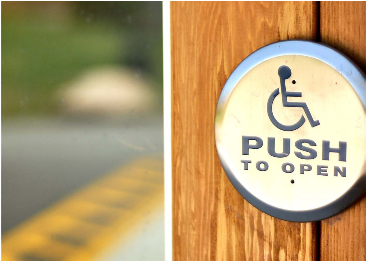
Push button for the barrier-free door operator at the new Curatorial Centre
